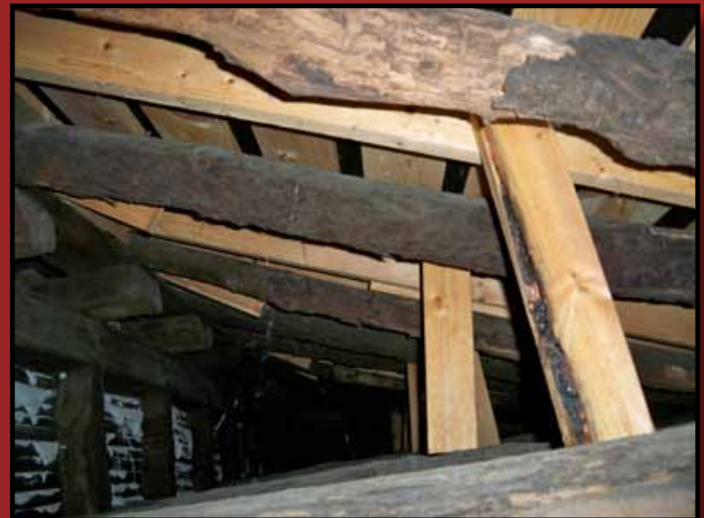
The original log beams are reinforced with new beams in the Shastid house roof.
